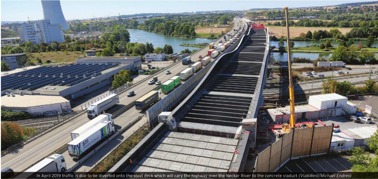
In April 2019 traffic is due to be diverted onto the steel deck which will carry the highway over the Neckar River to the concrete viaduct (Via6West/Michael Endres)
