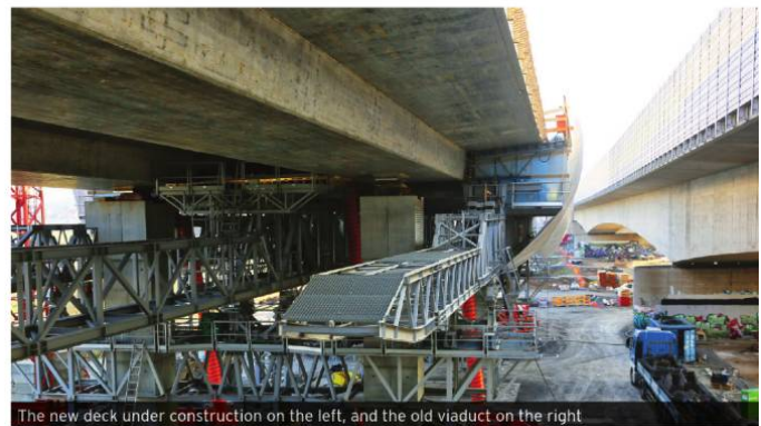
The new deck under construction on the left, and the old viaduct on the right
